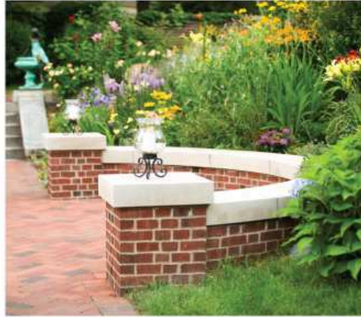
The limestone caps were difficult to acquire, but a necessity for restoration and complying with the Minnesota Historical Society.
